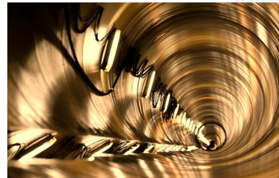
Transfer collectors for the Czajka waste water treatment plant in Warsaw (stage I)
