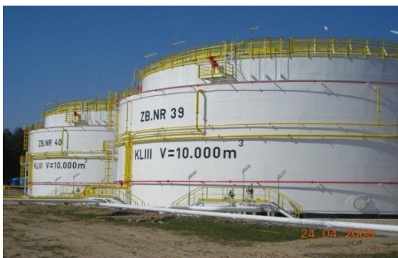
Storage containers in Rejowiec
